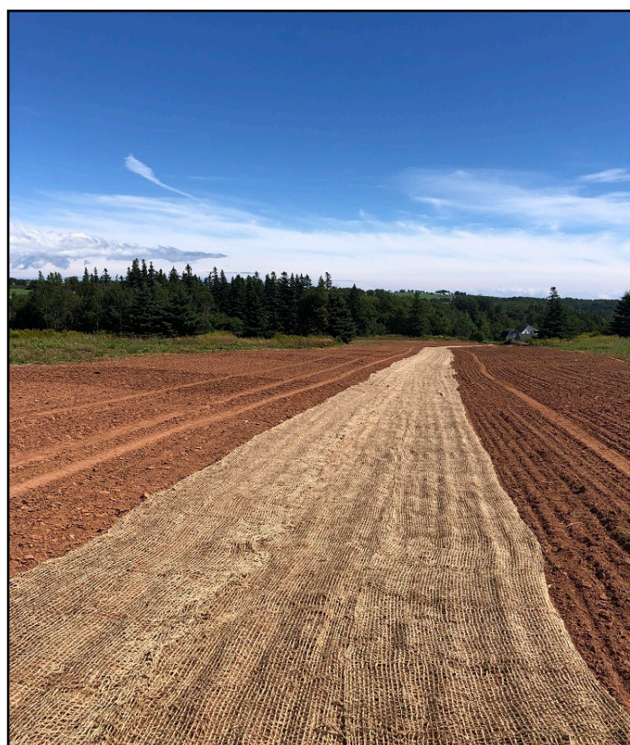
A grassed waterway on an AWP erosion control project. The jute mat was installed with the assistance of the local watershed group.
