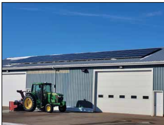
Shop Solar Panels
