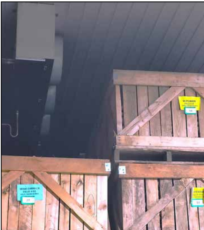
Field Warehouse Refrigeration
