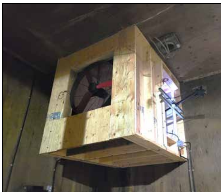
Walker Warehouse Ventilation
